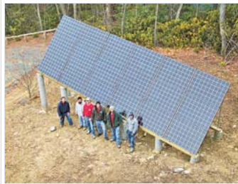
Al Lewis Construction is putting the finishing touches on a 30-foot by 12-foot solar power system from Weaverville's Sundance Power Systems in the backyard of a home on Green Hill Road in Blowing Rock. The Al Lewis Construction team is, from left to right, Joey Selby, Kenny Ward, Gary Sigmon, Al Lewis, Zack Spiegel and Dan Haigler. Photo by Sam Calhoun
