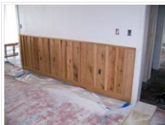
In addition to installing the solar power system, the Gaul family also remodeled the house reusing materials used in the original house. Contractor Al Lewis reclaimed oak from the former structure and reused it as the wainscoting in the remodel. Photo by Sam Calhoun
